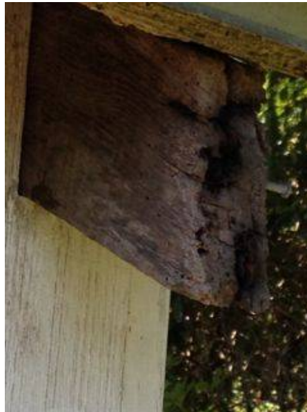
Photo 34-2 Rot and small insect holes on rafter tail.
