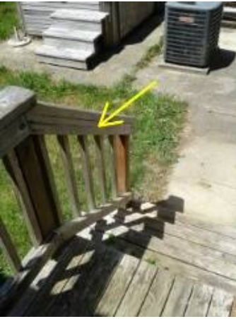
Photo 2-1 No hand grab on four riser stairs.
