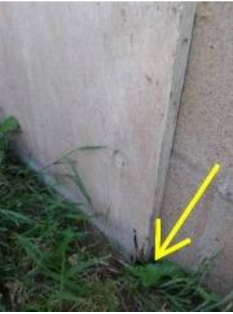
Photo 6-1 Crawl space access door in contact with ground. Wood to ground contact creates an environment conducive to wood destroying organisms.
