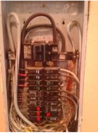
Photo 17-1 Main Electrical panel
