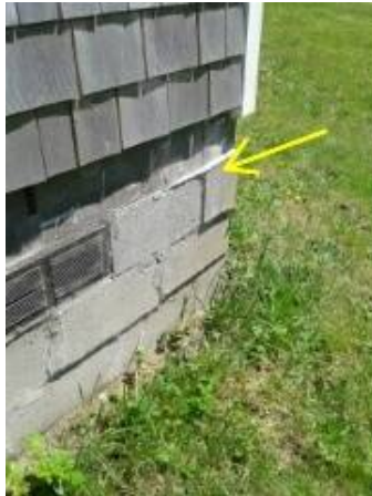
Photo 5-2 Poor workmanship in laying block foundation
