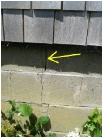
Photo 5-1 Crack in cinder block stem wall.
