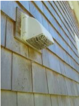
Photo 23-1 Dryer vent clogged and directly above propane tank.
