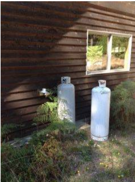
Photo 10-1 25 gallon propane tanks.
