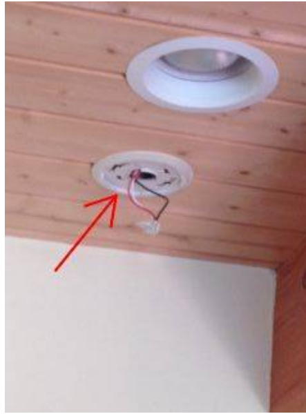
Photo 4-2 Disconnected smoke alarm
