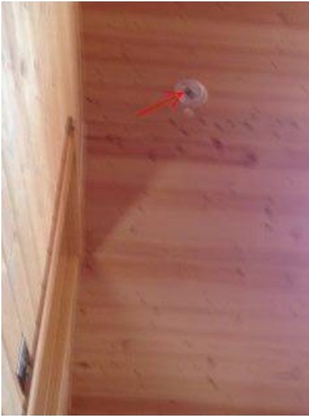
Photo 4-1 Disconnected smoke alarm
